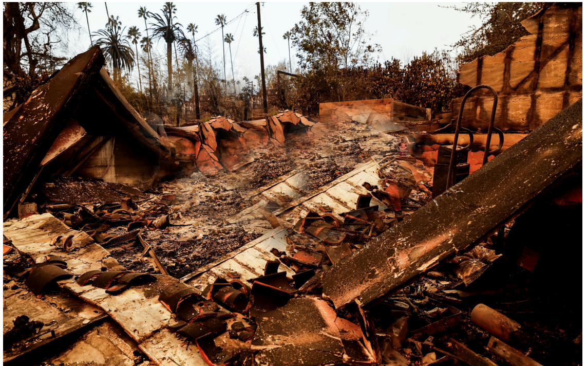
A burnt-down house stands in ruins, a stark reminder of the devastation caused by the Eaton Fire in Altadena, California. | This art was created with the assistance of Shutterstock AI tools
